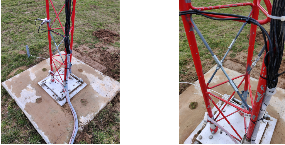
Figure 7.2: Photograph of the foundation and anchor plate (left), and photograph of the first bay and damage mechanisms in place (right).
