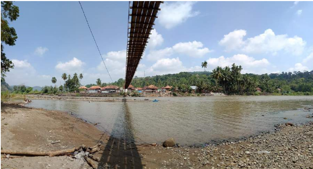
Temporary bridge is vital facility for people in Lubuk Sepang village, not only connecting it village with Perigi village, but also to the farms/fields around the villages
