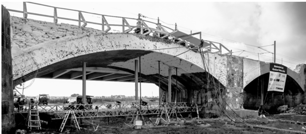
Figure 2. Side view from west of the arch 4 of the historic masonry arch bridge. The whitewashed area indicates the area of the direct influence of the load application. On the bridge: four hydraulic cylinders for the load application (Paffenholz et al. [27]). Reproduced with permission from Paffenholz, AVN; published by Wichmann-Verlag, 2018.
