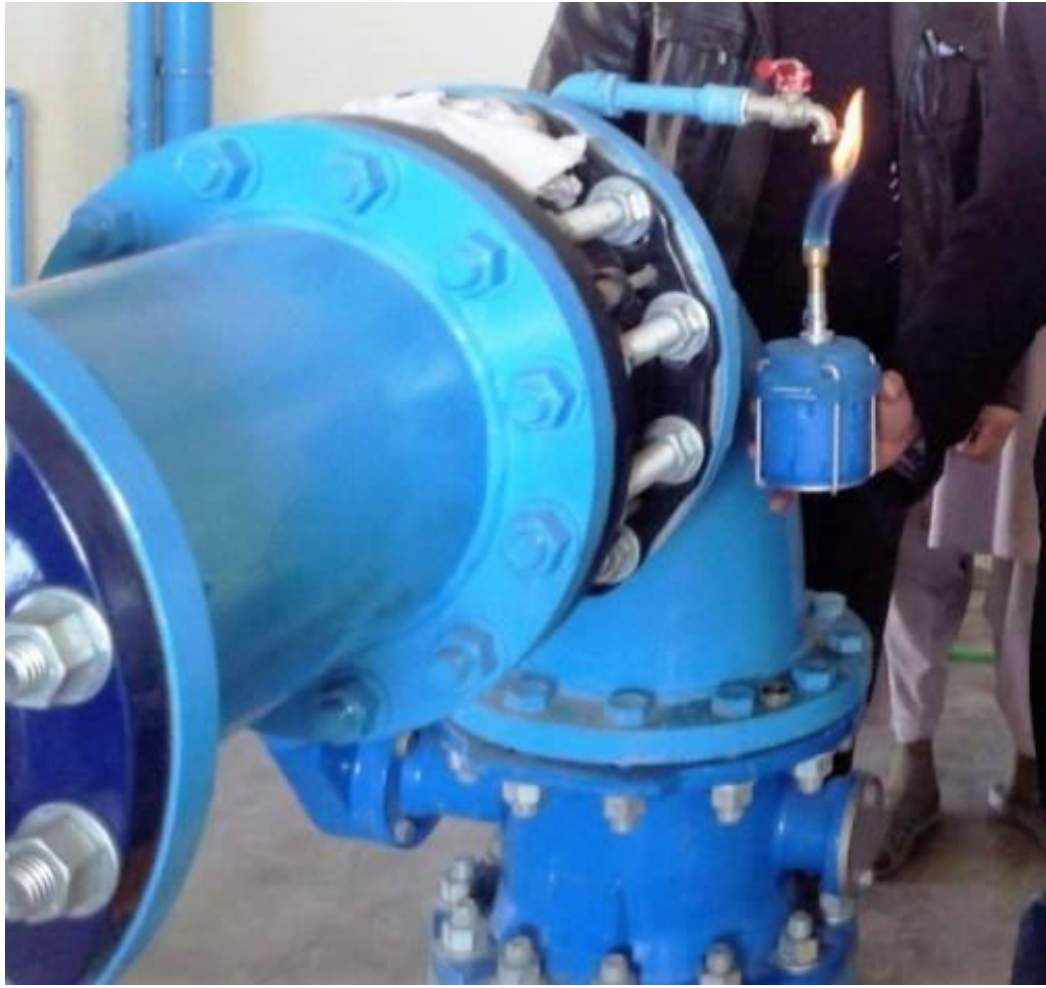
Fig.3.4: Heat sterilization of a water supply booster pump by a gas torch before sampling
