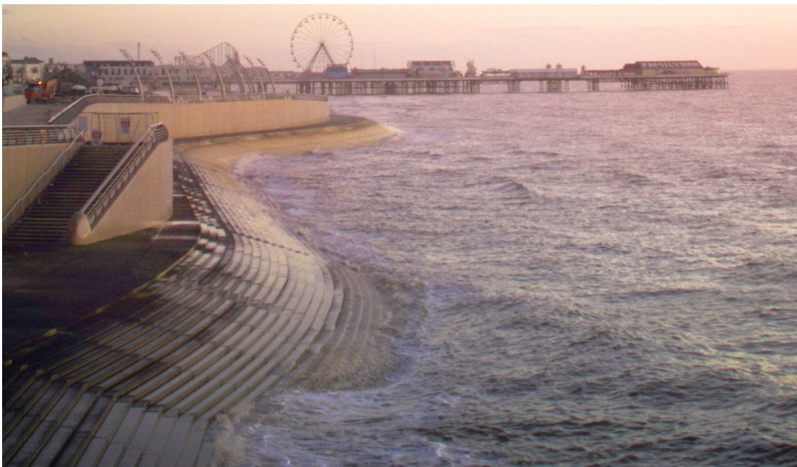
Figure 2.3: Blackpool revetment during high tide point to the fact of algae growth for areas with wet and dry cycles (photo taken from M. Beckwith in 2011).
