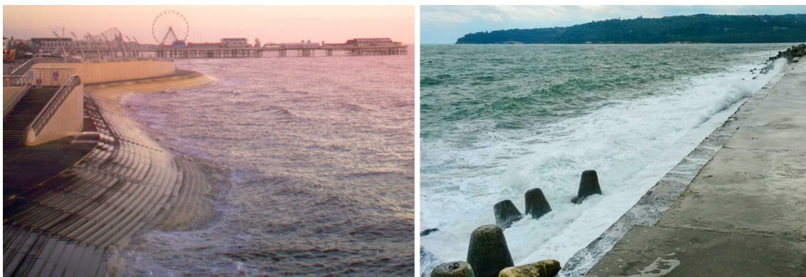
Figure 1.1: Examples of stepped revetments. Left: Shoreline revetment in Blackpool, UK (photo taken by M. Beckwith in 2011). Right: Stepped breakwater in Varna, Bulgaria in 2014.
