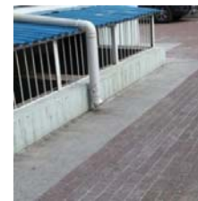
Figure 104: Drainpipe and permeable brick paving
