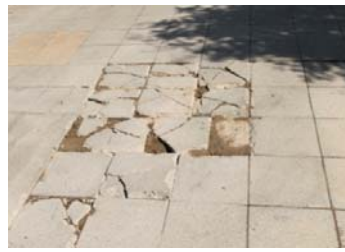
Figure 96: Damage to pavements
