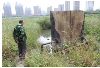
Figure 12: Pump station in the Park
