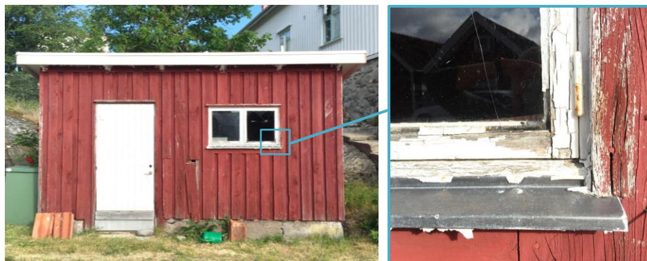
Figure 3: Wooden window with poorly maintained coating on a building in Kristineberg, Sweden. Defects in coating can cause enhanced water uptake due to capillary effects.
