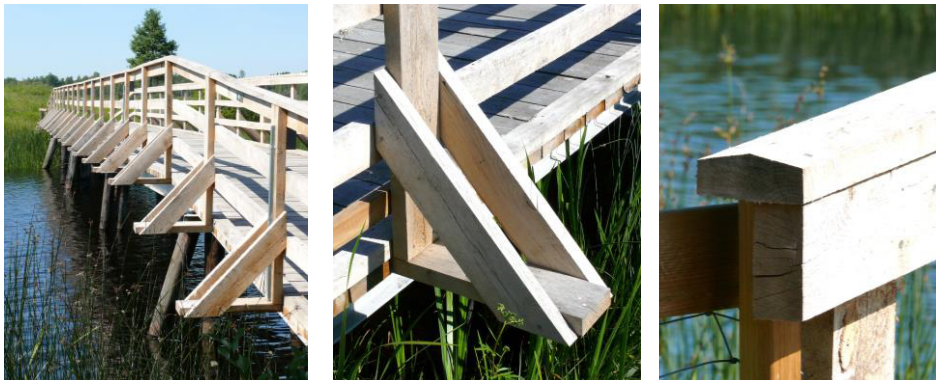
Figure 5: Bridge in Sävsjö, Sweden. Different design details causing water trapping and accumulation of moisture.
