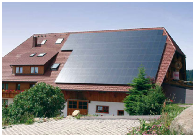
Figure 1.1: PV modules installed on a building roof. Picture taken from www.sunpower.de/haus/solarmodule-schwarz/ :30.12.2014
