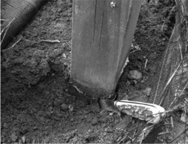
Figure 6. Failure of a fence post made from Douglas fir after only three years of exposure at the test site of the IBW in Hannover, Germany.
