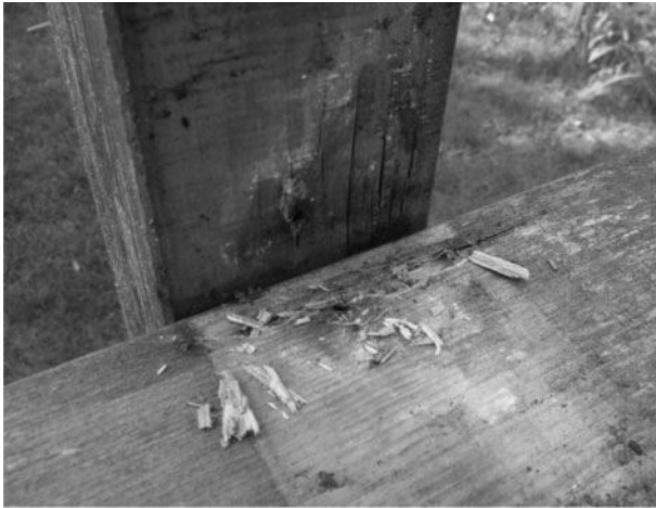
Figure 8. Severe decay caused by brown rot on the contact area of the picket and the post of a fence element made from Norway spruce after 4 years exposed at the test field of the IBW in Hannover, Germany.
