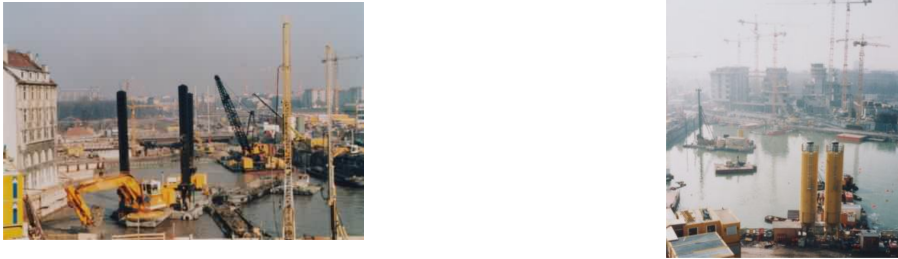
Figure 1.2: Picture of the Postdamer Platz during the construction showing pontoons on the groundwater table
