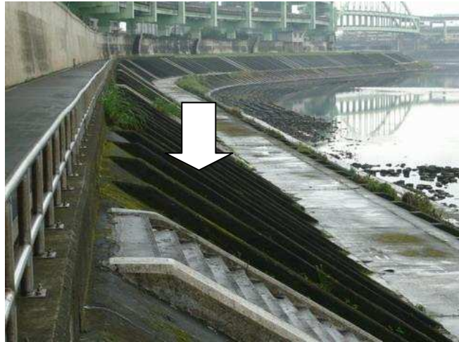
b. Location: along Nanhu Riverside Park, on the left side of Keelung River (L1040499)
