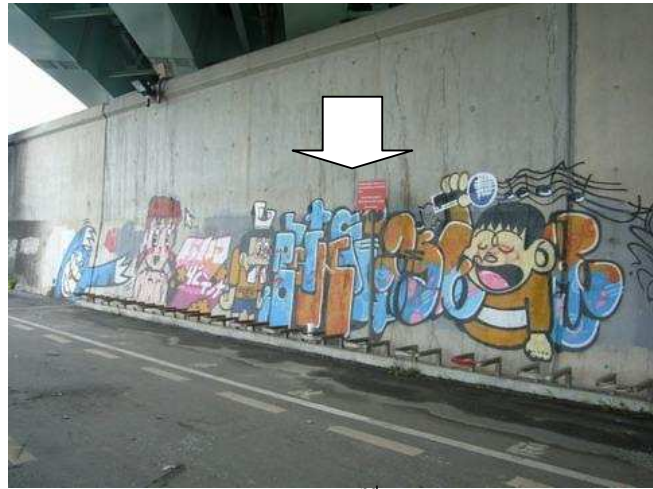
b. Location: under Maishuai 2 nd Bridge, on the left side of the Keelung River (L1040576)
