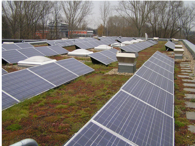
Fig. 3. On the roof of the maintenance depot Stammestraße a photovoltaic system was installed in addition to the roof greening. (DEPARTMENT ENVIRONMENT AND URBAN GREENSPACE, STATE CAPITAL HANNOVER)
