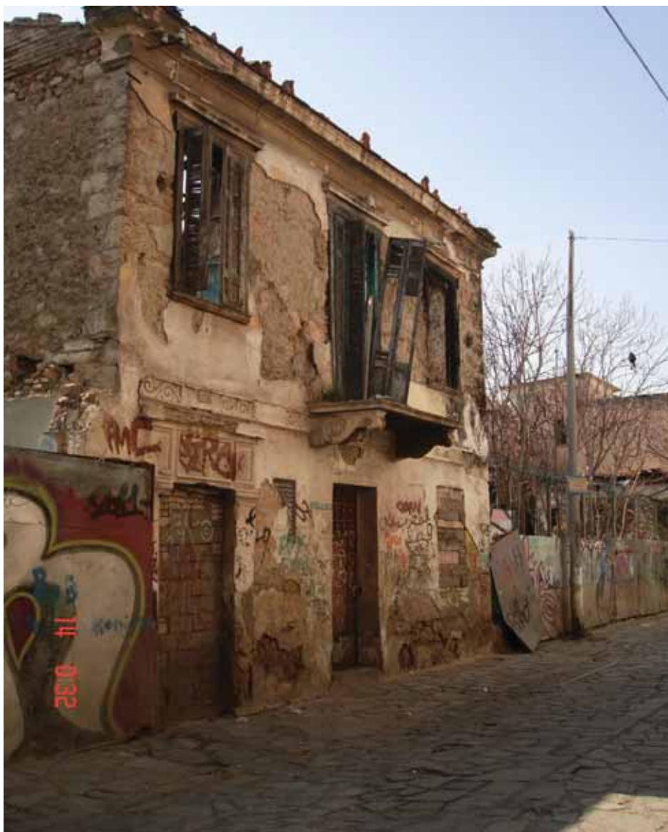
Figure 4: Problems of building maintenance at the heart of Athens. (Source: SAPOUNTZAKI 2014)
