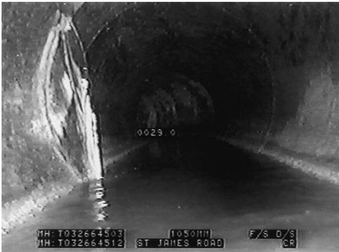
Figure 1.2: CCTV-image of a transversal crack-type pipe defect with groundwater infiltration. Reprinted from Davies et al. [2001].
