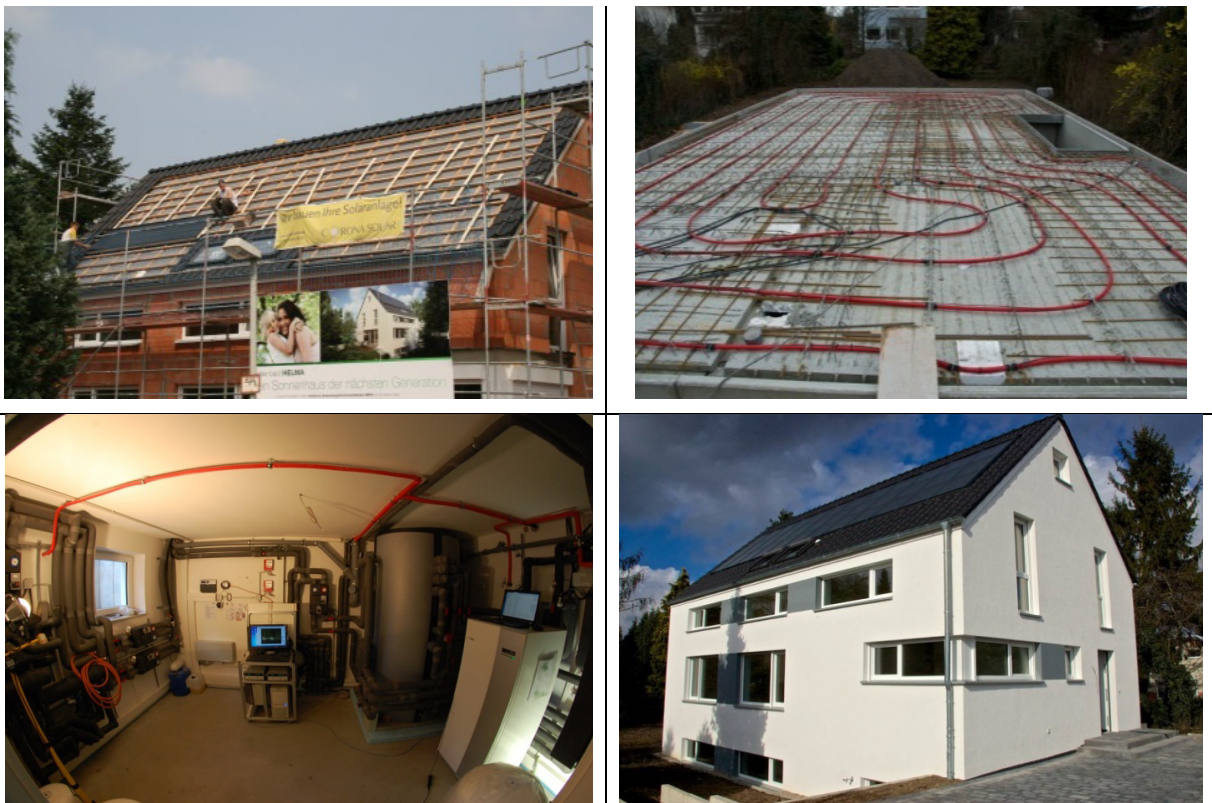
Fig. 5: Prototype building. Upper left: Implementation of solar thermal collectors, Upper right: Construction of thermal activation layer between cellar and ground floor, Lower left: Heating room after completion with data recording unit in the center, Lower right: Building after completion
