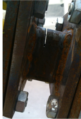
(b) Damage imposed to one of the braces
