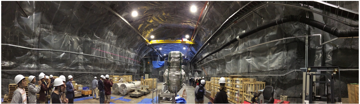
Figure 2.9: KAGRA under construction. This panorama photo was taken in June 2014 when I was visiting KAGRA which is located underneath a mountain near Kamioka.
