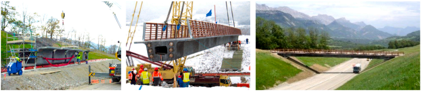
Fig. 2. Bridge PS34: assembly of the 22 UHPFRC segments with 12.0 cm wall thickness and keyed dry joints next to the highway (left) [14], lifting of the 47.7 m long superstructure with only one truck-mounted crane (middle) [15] and finalized bridge (right). Source: C. Clergue
