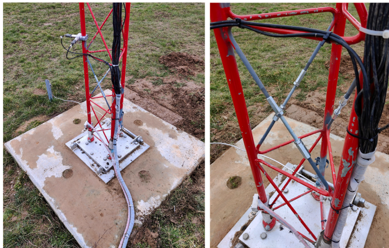
Fig. 8. Photograph of the concrete foundation (left), and the reversible damage mechanisms at level 6 (right) [34].
