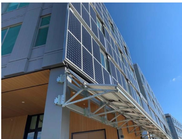
Figure 14. Traditional solar in place of metal cladding on Colorado’s first net-zero multi-tenant building Boulder Commons, Boulder, CO. Photo courtesy of Christopher Klinga.
