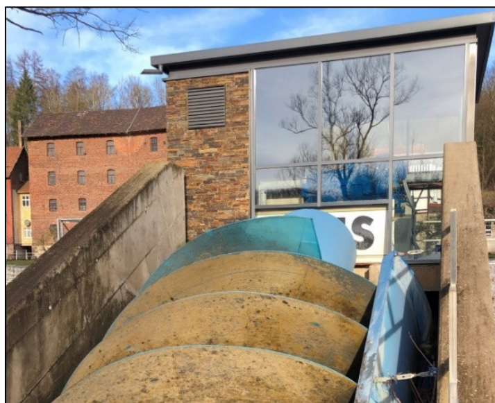
Figure 23. Hydraulic screw installed on the premises of a brewery in central Germany (photo by J. Dietrich).
