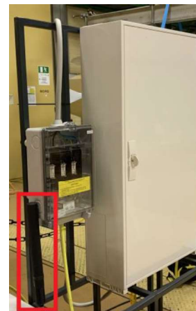
Figure 9. Omnidirectional antenna adjacent to consumer unit.
