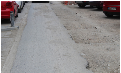
Fig. 3: Severe street damage on the Vakchou road (JELLE SCHACHT, 2023)
