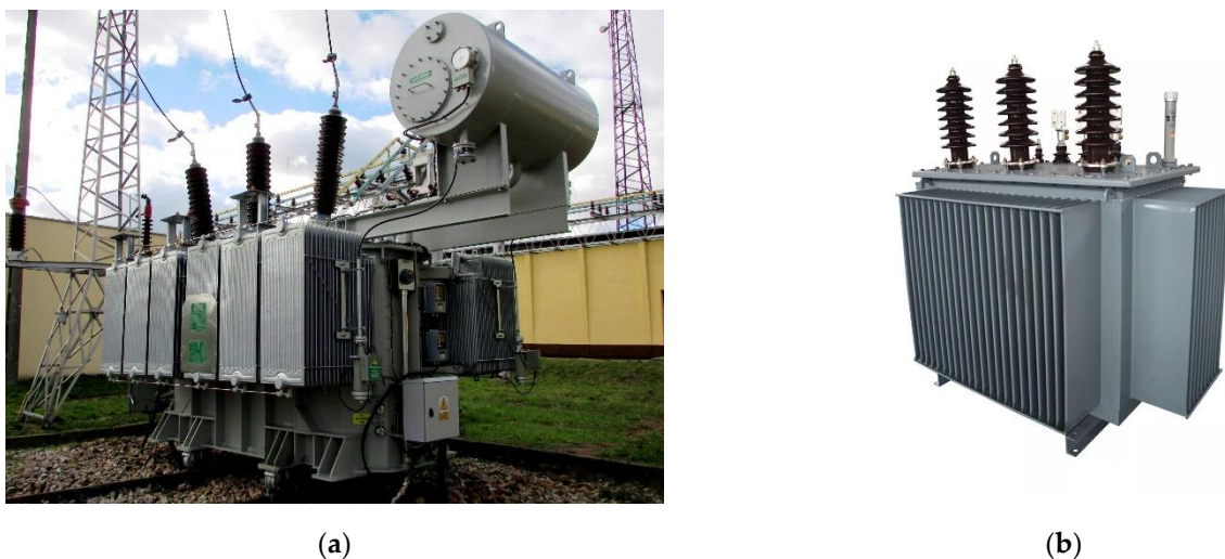
Figure 1. Application of liquid-paper insulations in power transformers: (a) Free breathing power transformer [25]; (b) Hermetic transformer [26].
