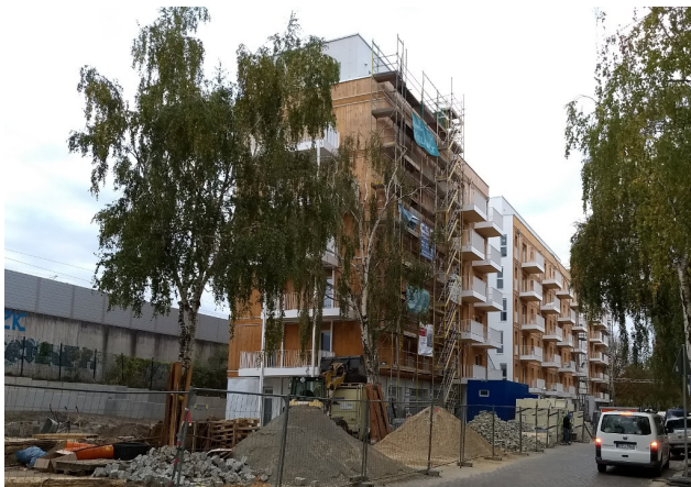
Figure 6: Photograph of the timber building and the railway embankment in Berlin, Germany.
