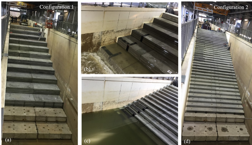
Figure 5.2: Stepped revetment model setup (cot \alpha = 3 ). (a) Configuration 1 with step heights of 0.50 m during construction and (b) model testing. (c) The small steps of (d) Configuration 2 with step heights of 0.17 m.
