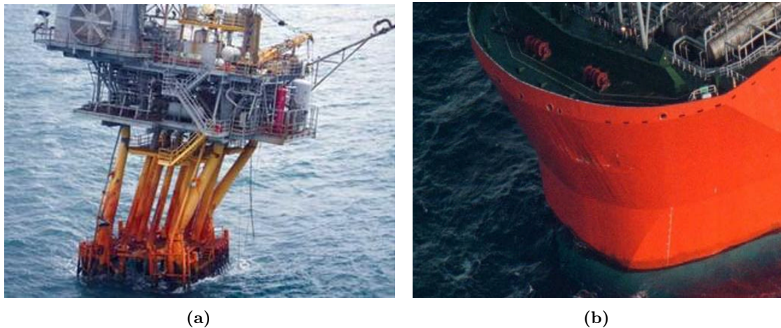
Figure 1.3: Wave slamming damage examples (a) on a platform in Gulf of Mexico during Hurricane Ike (taken from https://www.offshore-mag.com ), and (b) on a FPSO (taken from Buchner et al. (2004)).
