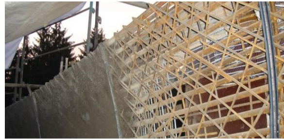
Figure 2: Shotcrete method used for the construction of the bobsleigh run in Oberhof [Torkret GmbH]
