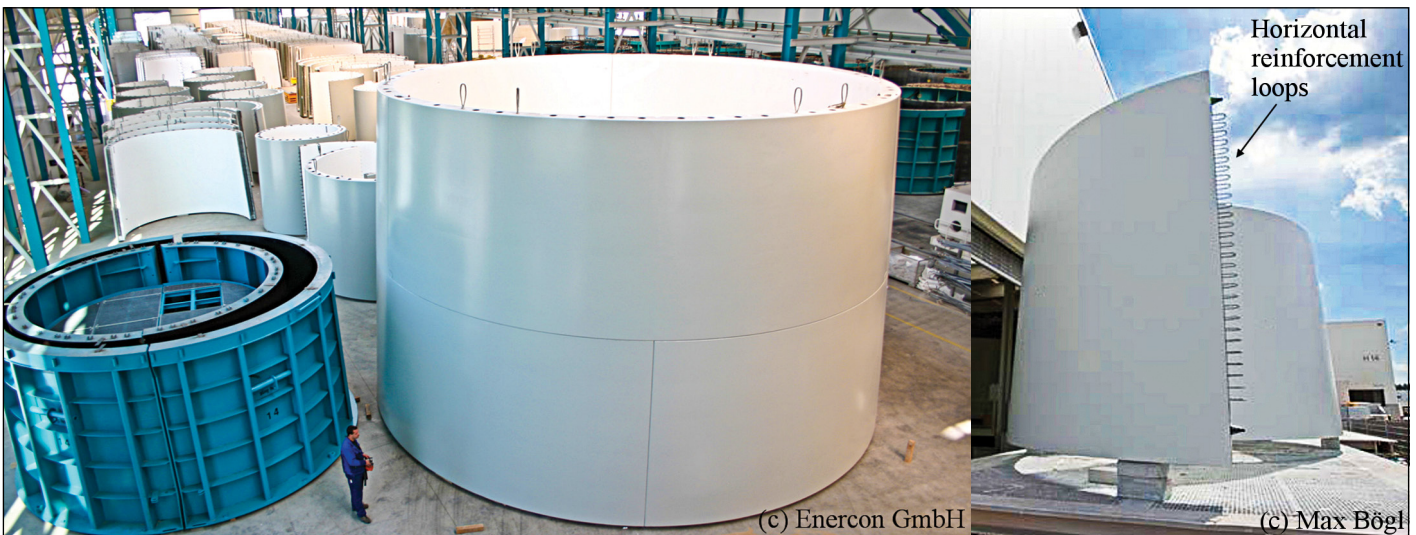
Figure 2 Precast plant for precast concrete segments (left) and horizontal reinforcement loops of a precast concrete segment (right)
