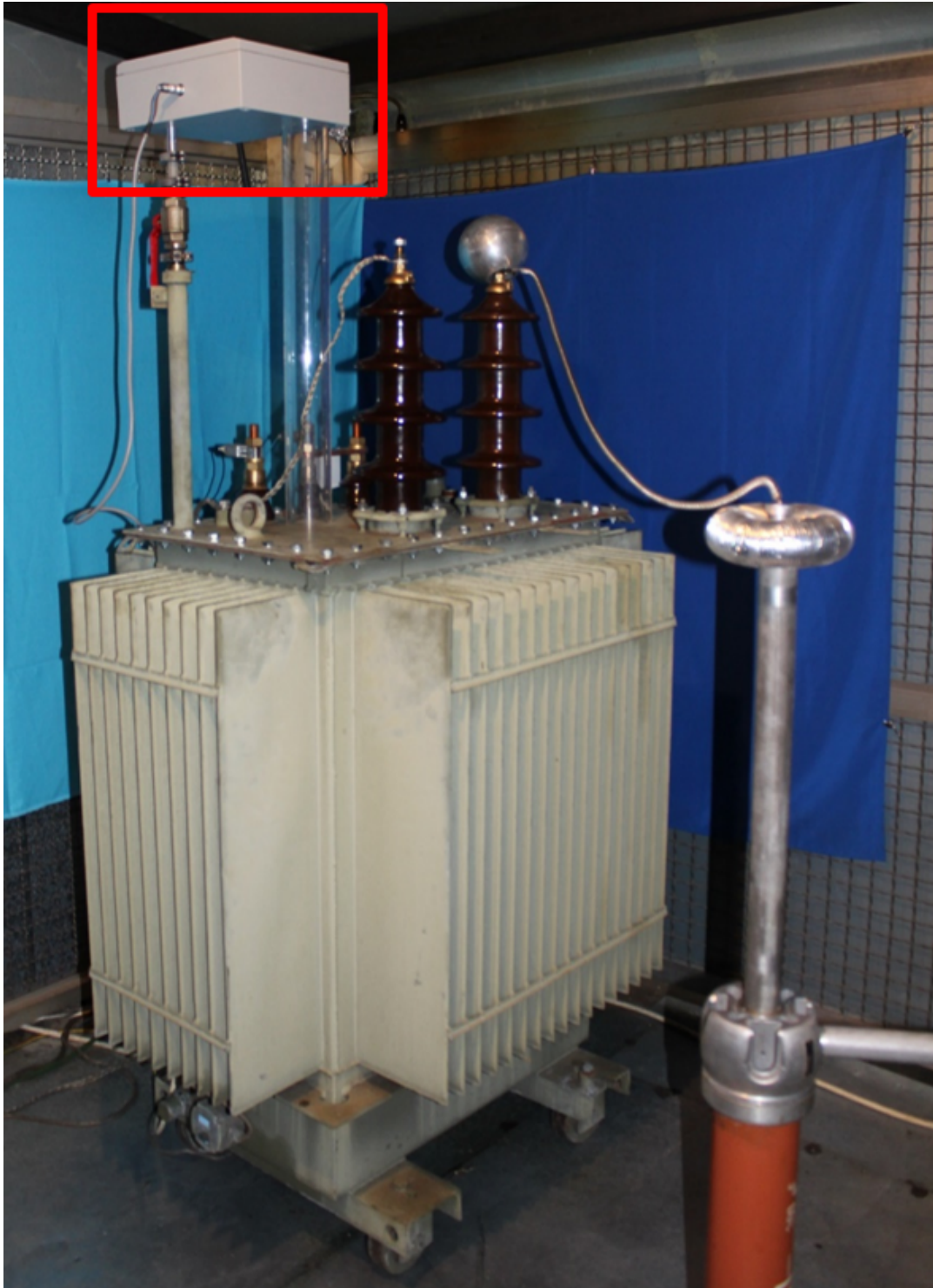
Figure 2.22: The hermetically sealed transformer with the installed lab prototype on the oil filling pipe [144]
