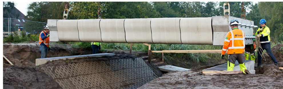
Figure 5. The 3D concrete printed pedestrian and bicycle bridge in Gemert, the Netherlands, is hoisted into position. Reprinted with permission from ref. [3]. Copyright 2018 Cement and Concrete Research.
