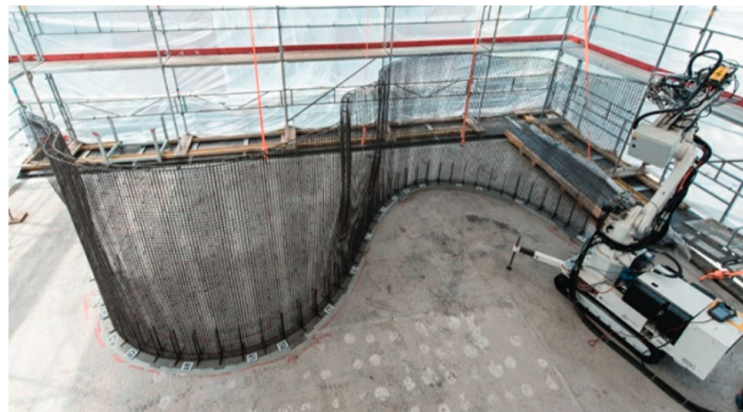
Figure 4. Production of 14 m long mesh for a double curved load-bearing wall for the DFAB HOUSE, Switzerland. Reprinted with permission from ref. [49]. Copyright 2018 Cement and Concrete Research.
