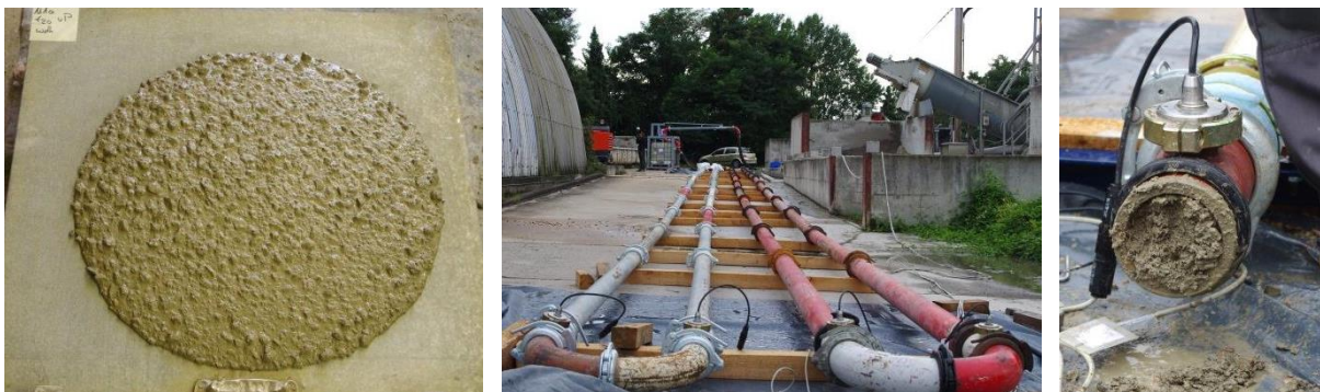
Figure 1.3: Blockage of pumping line (Research project: TUD and LUH)
