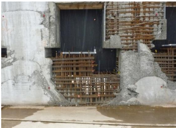
Figure 1.2: Pitfalls of conventional concrete with dense reinforcements [7]
