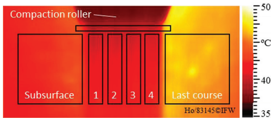
Fig. 1. Thermal process image within the ROI.
