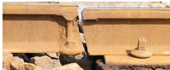
Figure 6. Broken rail joint [10]. (The image is licensed under the Creative Commons Attribution-Share Alike 3.0 Unported license.)
