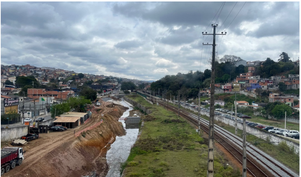
Figure 93 - Infrastructure works to reduce flooding along the Juqueri River around the Baltazar Fidelis train station in Franco da Rocha. Source: author's own collection
