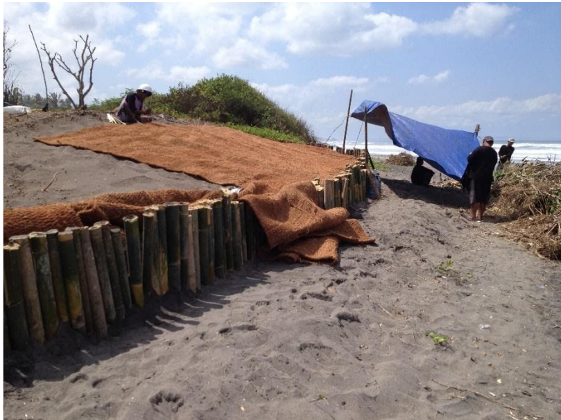
Fig. 8 Pictures of the on-site coir geotextile installation. The upper picture shows the cross-sectional view on the textiles. The bottom picture shows the bamboo wall and the installation of the top coir layer. © David 2014
